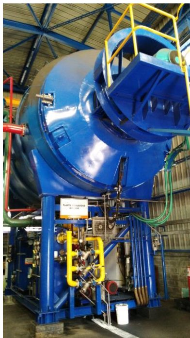
Desalination Plant MCV 500
