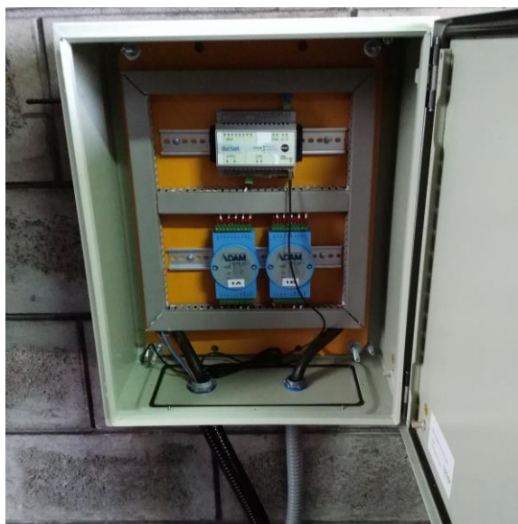
Hardware plant / platform interface
